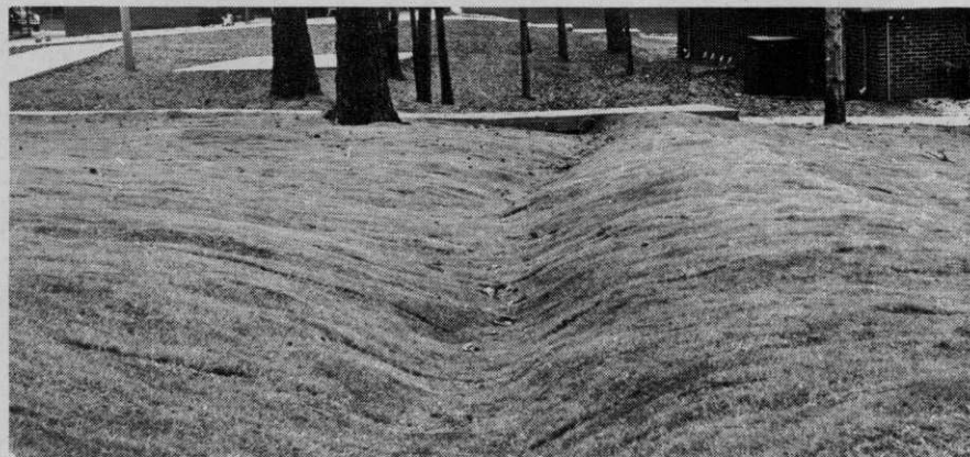
7. Trees, sidewalks and ditches presented no problem on this job which was laid by an inexperienced crew.
