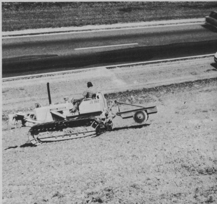
Mulch anchoring tool for incorporation of seed and mulch with soil requires heavy power unit. Work was done on the John F. Kennedy Memorial Highway in the state of Maryland. Effort was a government research project in cooperation with state.
