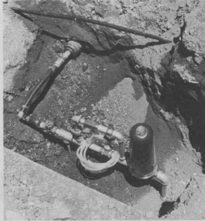
A filter and fertilizer applicator can be integral part of the system.
