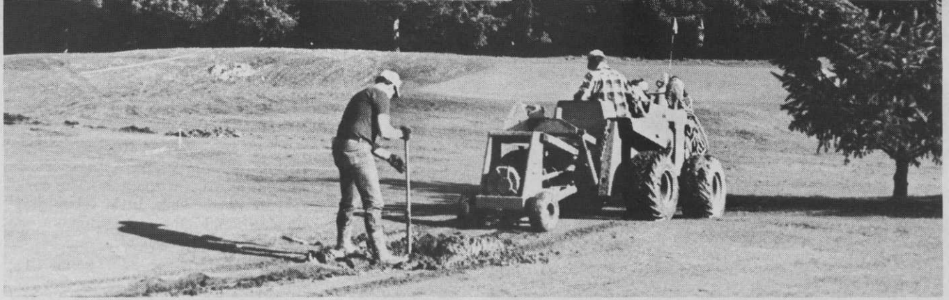
The R60 Ditch Witch with vibratory plow attachment installs plastic pipe for underground sprinkler system without digging a trench. The procedure begins by digging a hole in the ground.
