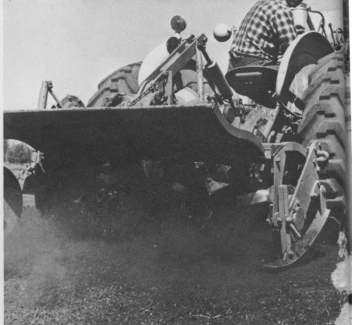
The sand-bark process calls for rotovating the sand and bark to a two-to-one mixture for a depth of eight inches. The construction method was developed by landscape architect Ellis Van Gorder.
