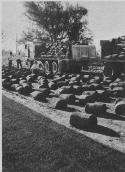
Sod is loaded on trailer trucks for installation by Cloverdale crew at landscaping site.
