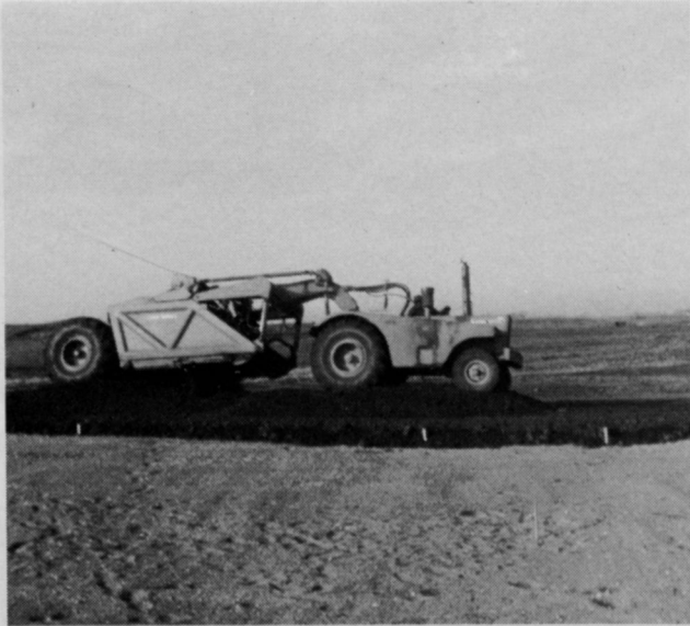
Equipment such as this used at Jesup, Ia., course is practical for moving and handling topsoil mix.
