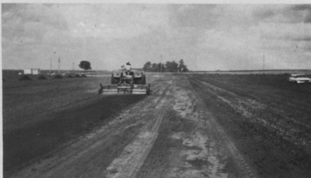
Step 1. Roto-tilling soil in 20-foot strips permits equipment to work on both sides without compacting. Soil has previously been spread to rough 4-inch depth by grading.
