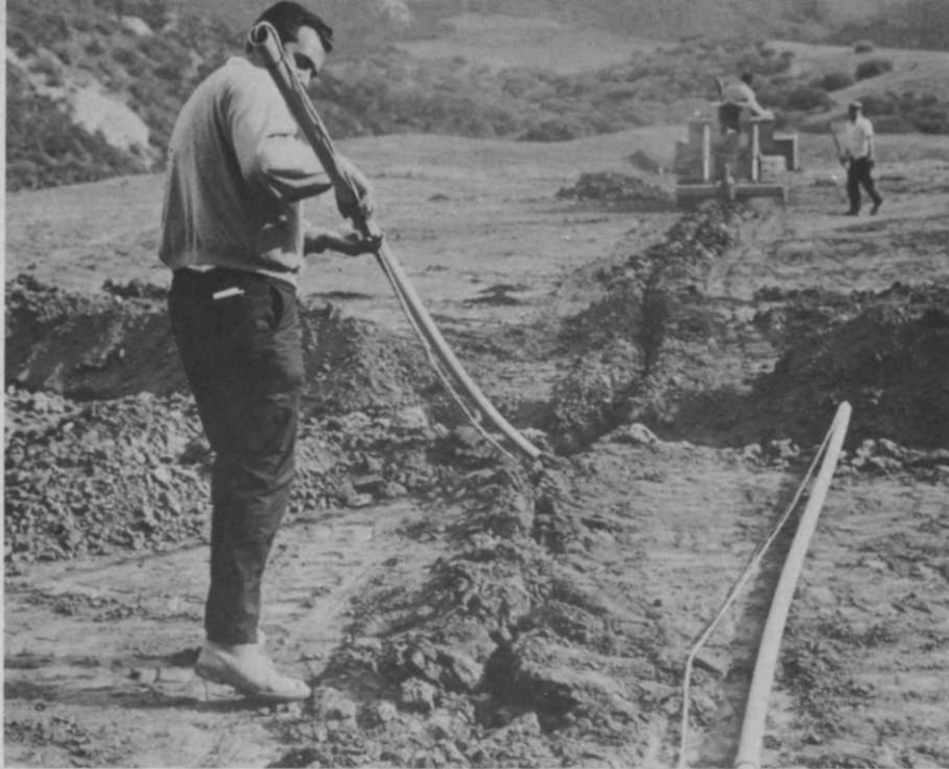
Laying 1½ inch pipe during installation of Calabasas Golf Course. Contract for entire course design, construction, and irrigation totaled more than $350,000.
