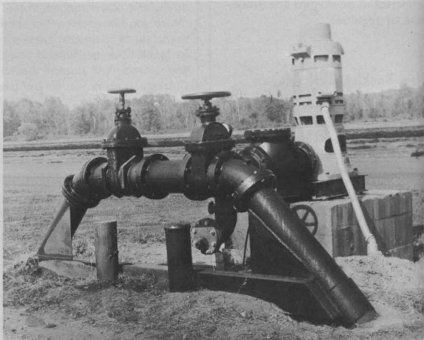
Electrically driven deep well pump is one of 3 used at Emerald Valley Turf Nurseries. Pumps can deliver irrigation water at rate of 2½ million gallons daily. Four miles of 10-inch underground pipe is used to carry supply to quick-coupling surface pipe.
