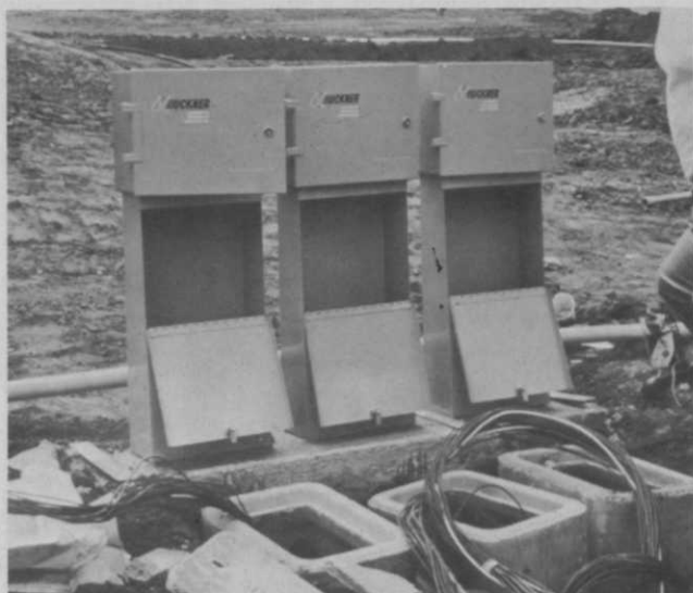
More than 100 miles of control wire was laid to provide the automatic control between pressure regulator control valves and controllers.
