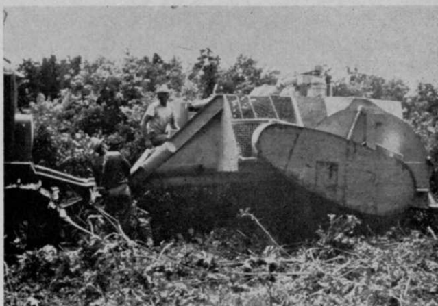
Company built flail unit for use by maintenance crew is used to clear right-of-way of brush growth. Unit is pulled by crawler tractor.
