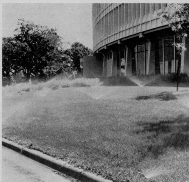
Underground automatic watering system permits flexibility required for efficient operation. Watering practices based on grass needs and keyed to existing soil and climatic conditions assure high quality turfgrass, necessary for maintaining green color throughout season.
