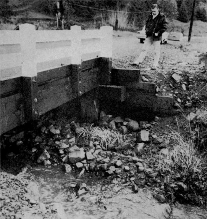
Bridge abutments, culverts, sign posts, and similar areas previously inaccessible to power equipment are easily covered with chemical spray equipment. Lane County costs approximate 63¢ per structure to spray.
