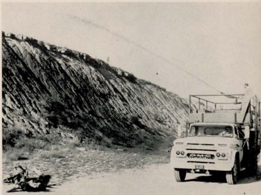
Conwed Hydro Mulch is being applied in this instance to a typical slope by hydraulic method. Seed, mulch and fertilizer are mixed, then applied on soil at distances up to 100 ft.
