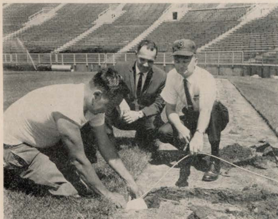
King-sized "heating pad" installed at Lambeau Field, home of the World Champion Green Bay Packers, will keep turf soft and frost-free during late season games. Checking the installation are left to right, Elmer Cloud, installer, Sal Soscia, application engineer for General Electric Company's wiring device department which supplied the cable, and George Halas, General Electric sales engineer. The cable, 14 miles long, covers 73,000 square feet of the Packers' playing field. Power required to "heat" the turf is equivalent to that needed to light 7,800 100-watt bulbs. Halas is an occasional scout for both football leagues and a nephew of George "Papa Bear" Halas, owner and coach of the Chicago Bears.
