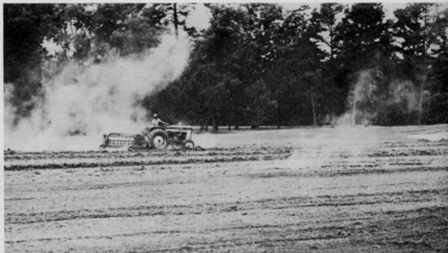
Raking up old turf on fairway, Southern Turf crewman readies soil for replanting new grass.
