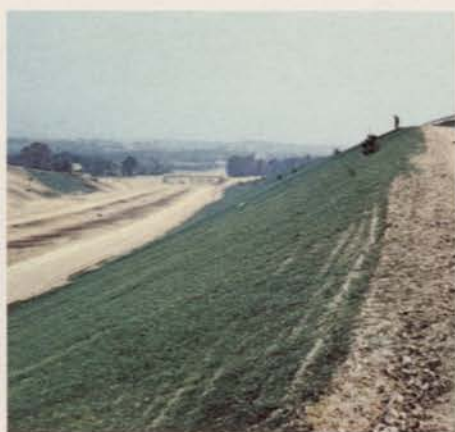
2. Here's the same slope several weeks later. Adjacent slopes seeded the same day by conventional straw method had a much poorer stand of grass and considerably more erosion.
