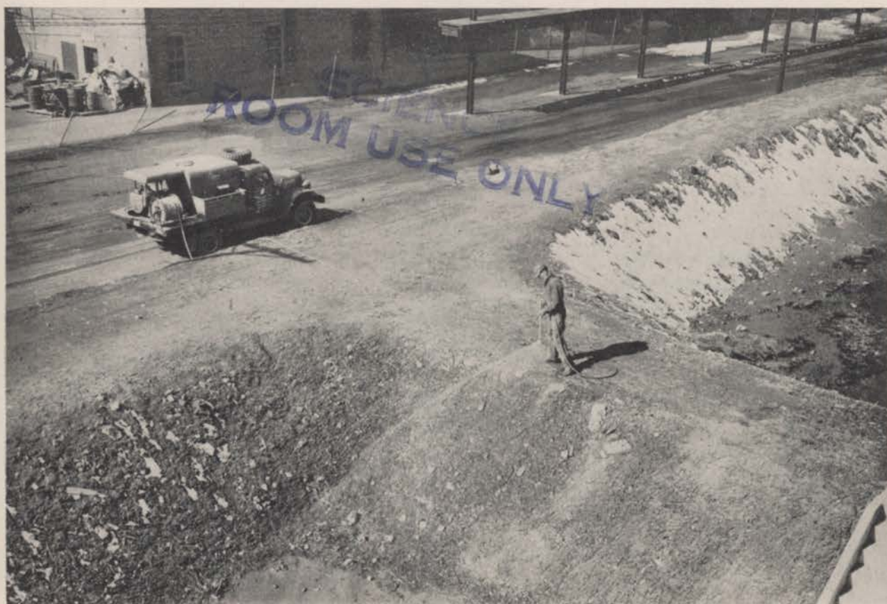
Contract sprayer on soil sterilization job on roadways inside an industrial establishment.
