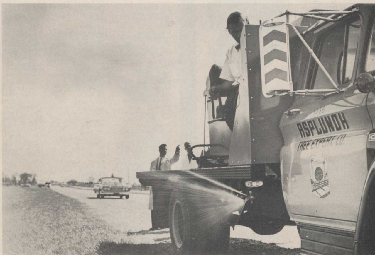
Typical contract sprayer on highway job. Asplundh had this spray rig especially built by the John Bean Division, FMC Corp.
