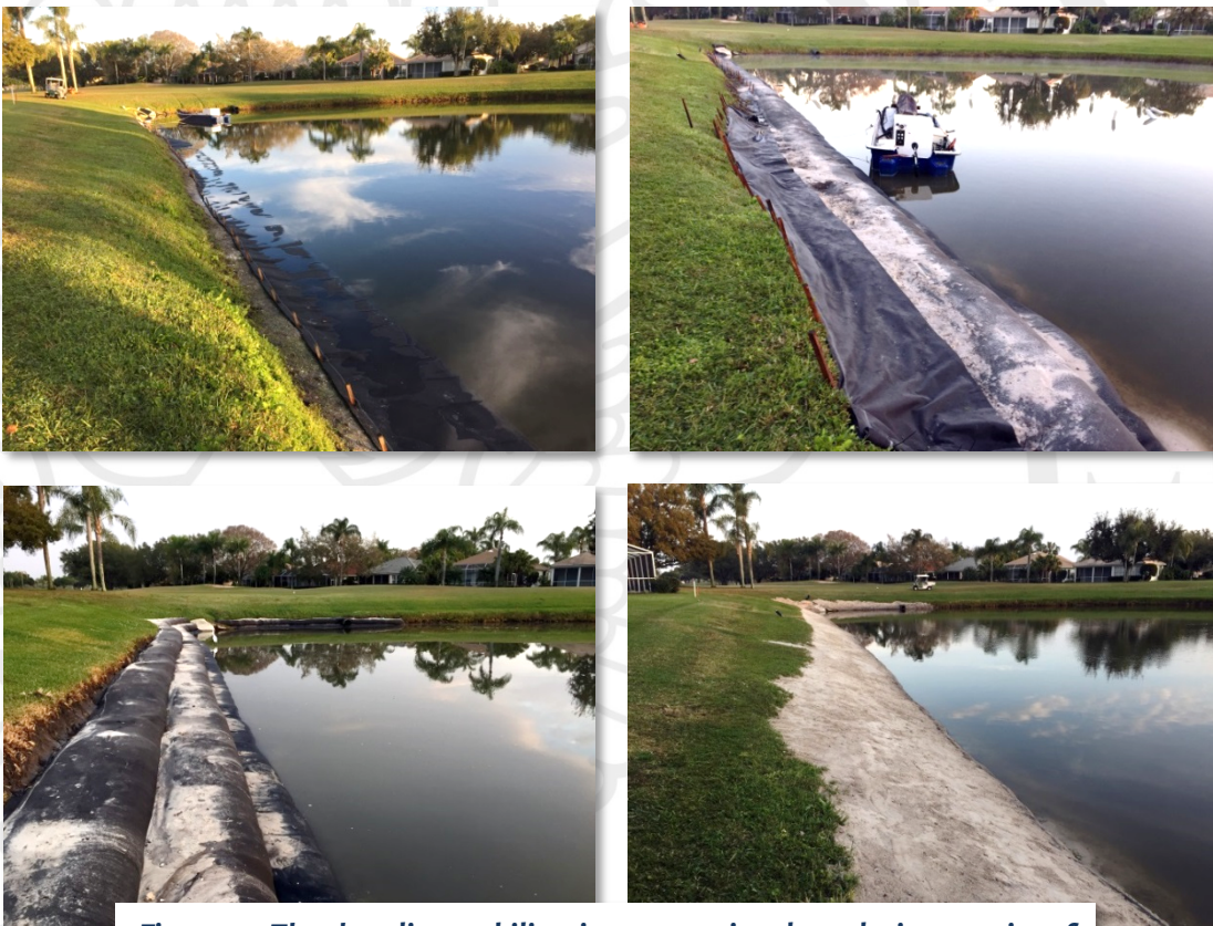
Figure 2 - The shoreline stabilization process involves placing a series of geotextile tubes along the shoreline (upper left), filling them with sediment from the bottom of the pond (upper right, lower left), covering the tubes with soil (lower right) and eventually sodding the slope.
