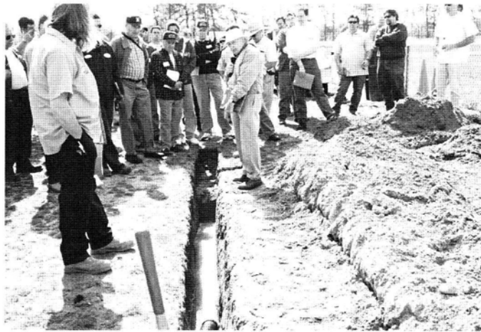
Dr. Henry Inkyk, SFMANJ Advisor and GSI Sports Field Consultant describes the steps in installing drainage.
