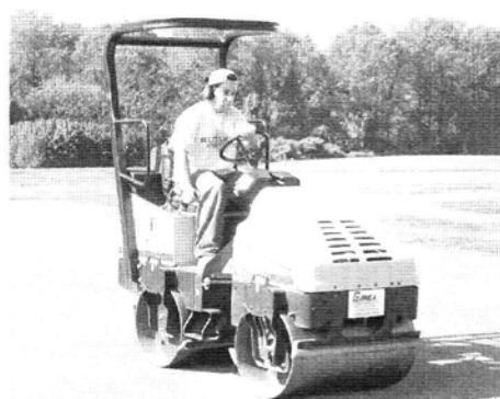
Figure 2. A roller (2970 lbs) was used to create compaction in the test plots.
