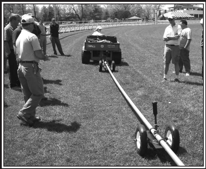
The complexities of irrigating Monmouth Park's oval-shaped thoroughbred turf track and a fixed inside rail necessitate the use of an innovative towline irrigation system.
