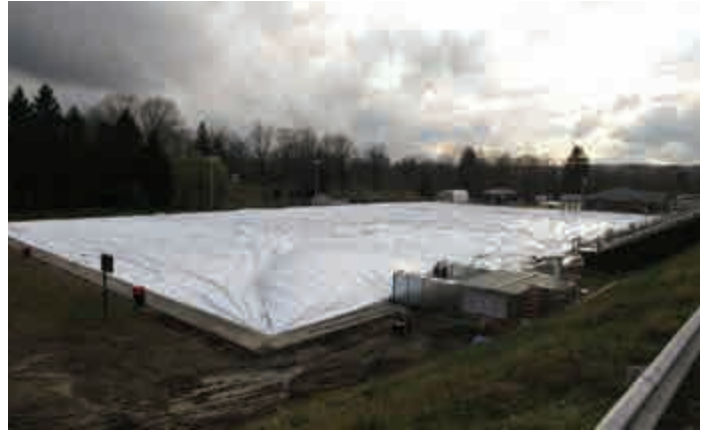
Dome spread out and connected to the grade beam, beginning inflation (Greenville, PA).
