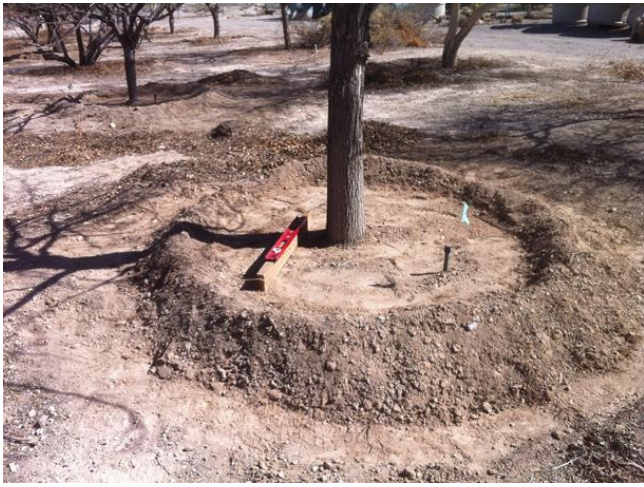
Basins built around each tree to hold irrigation water
