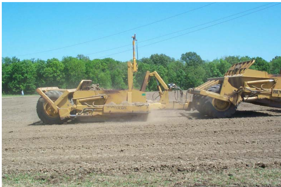
In April, 2003, approximately 2.5 acres of land at the Blackbelt Experiment Station located at Brooksville, MS was laser-leveled to obtain a slope of 3% having no measurable cross-slope.
