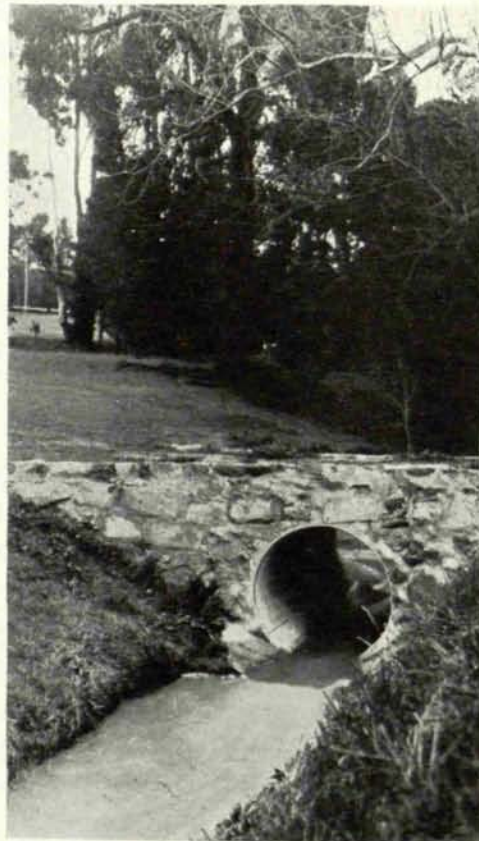
THIS SMALL STREAM ON THE CLAREMONT COUNTRY CLUB OF OAKLAND, CALIFORNIA, IS CROSSED BY A CORRUGATED IRON CULVERT BRIDGE. Stone masonry head walls give a rustic appearance that harmonizes with the immediate surroundings
