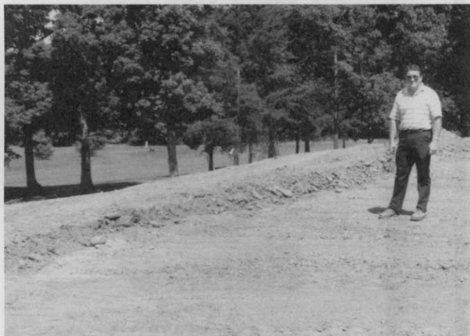
Steve Nash examines an excavated bunker. In addition to the greens construction, Steve and his crew are building two new tees and two fairway bunkers.
