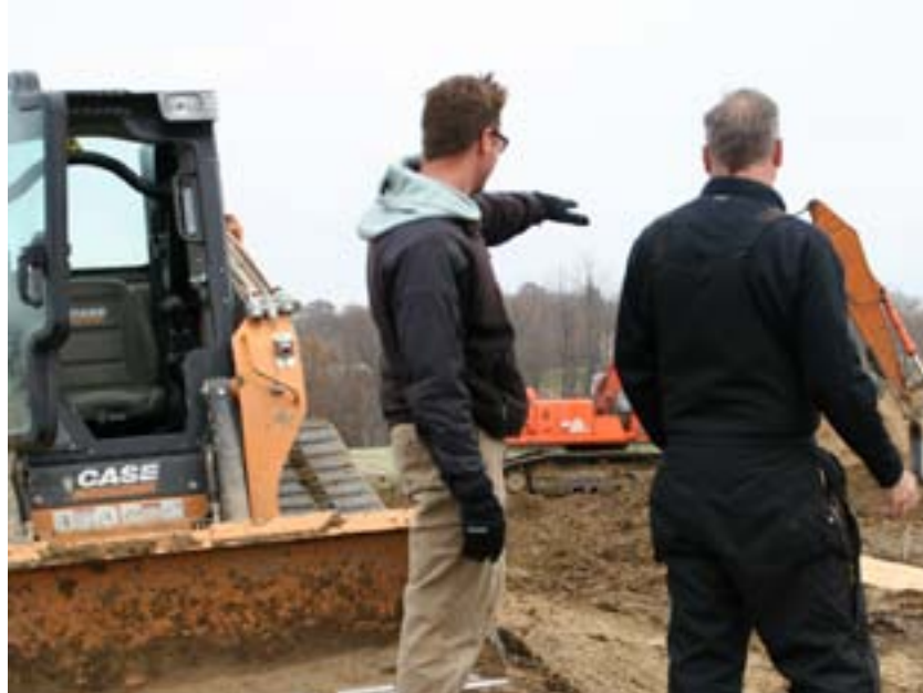
Hines and First Assistant Todd Kranz review a construction project taking place at Windsong Farm.
