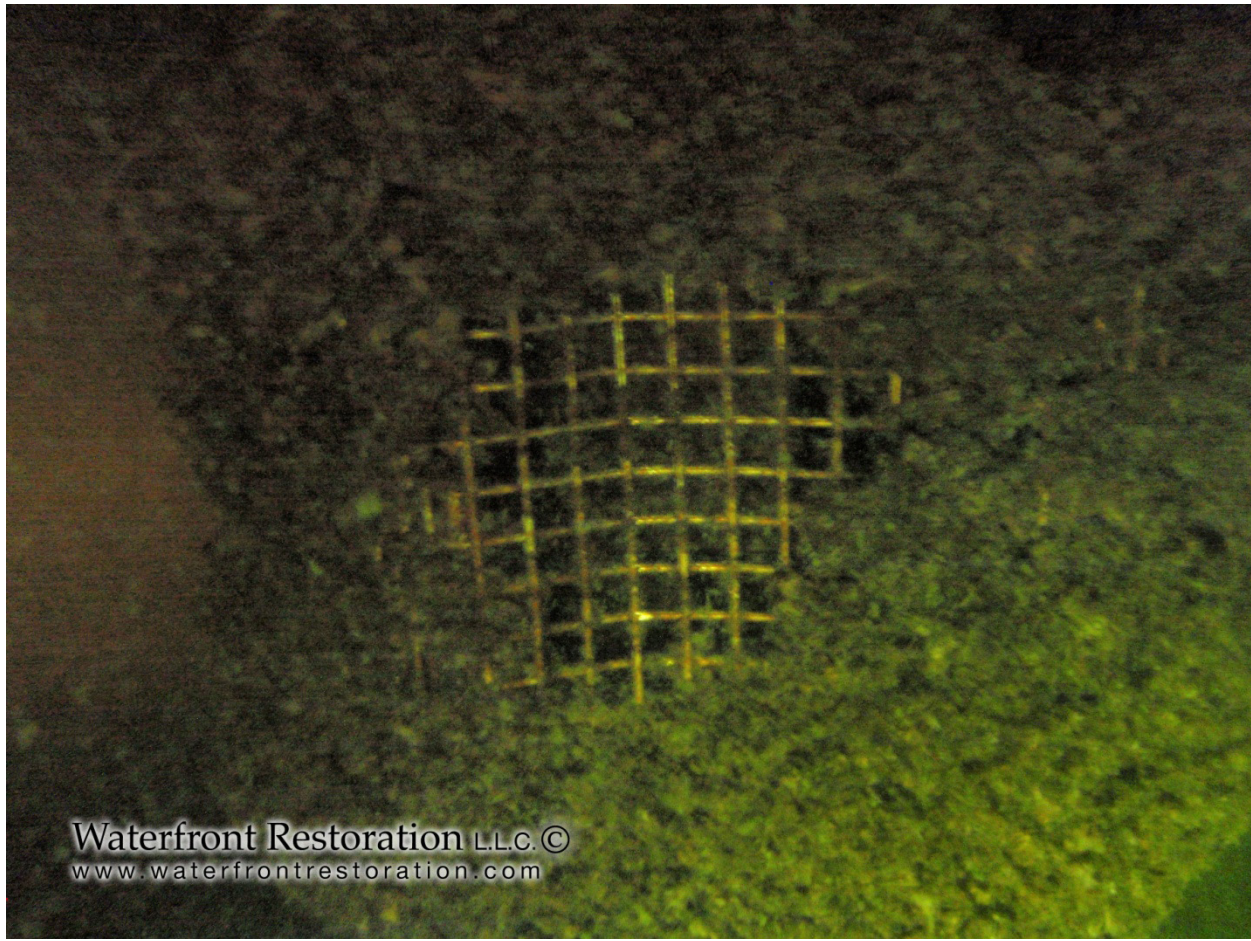
Intake1 heavily covered in zebra mussel buildup, causing significant obstruction of water flow
