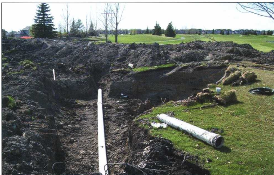
Irrigation repair was a consequence of the flood.
