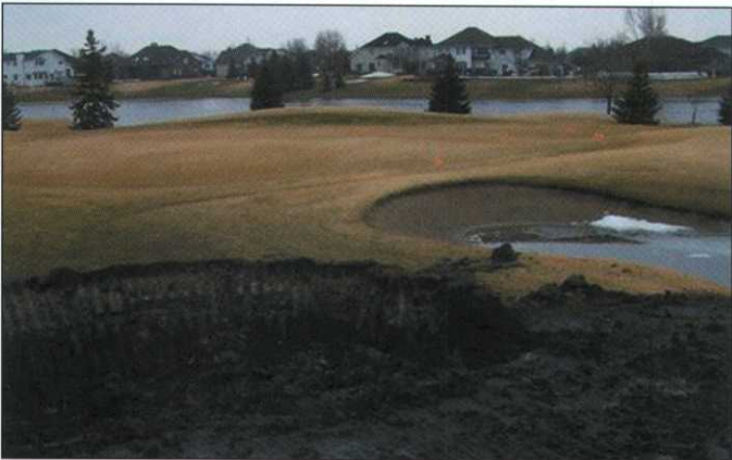
Parts of the course were disturbed in order to build the dikes.
