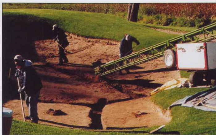
Using the conveyor to empty the bunker.
