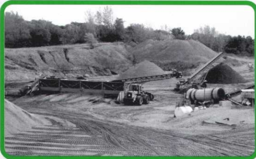
Blending yard with blender, stacking conveyor and stock piles.
