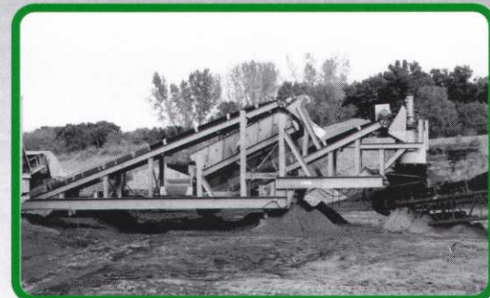
Screen deck and stacking conveyor.
