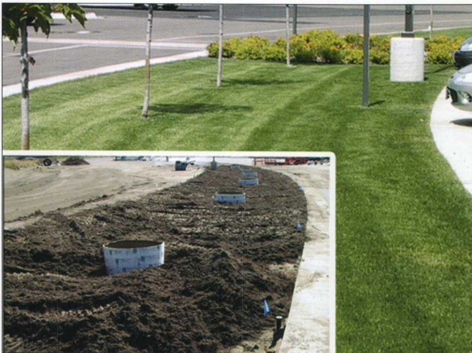
Before and after installation of the Netlon Advanced Turf rootzone. Profile consists of the right rock, sand, and amendments (peat and mesh) to provide maximum infiltration and stability.
