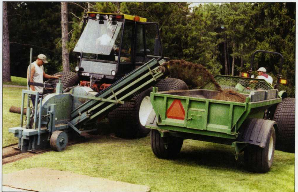
FAST AND QUICK. The Shelton Super Trencher cuts a trench up to 5" wide and conveys it away to the removal cart.
