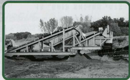
Screen deck and stacking conveyor.
