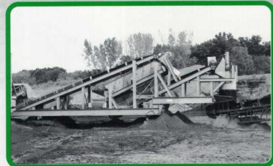
Screen deck and stacking conveyor.
