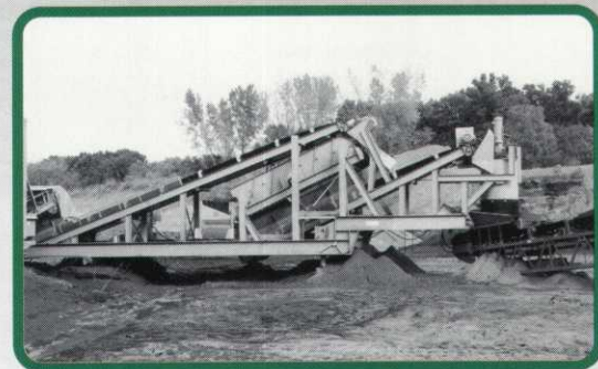
Screen deck and stacking conveyor.
