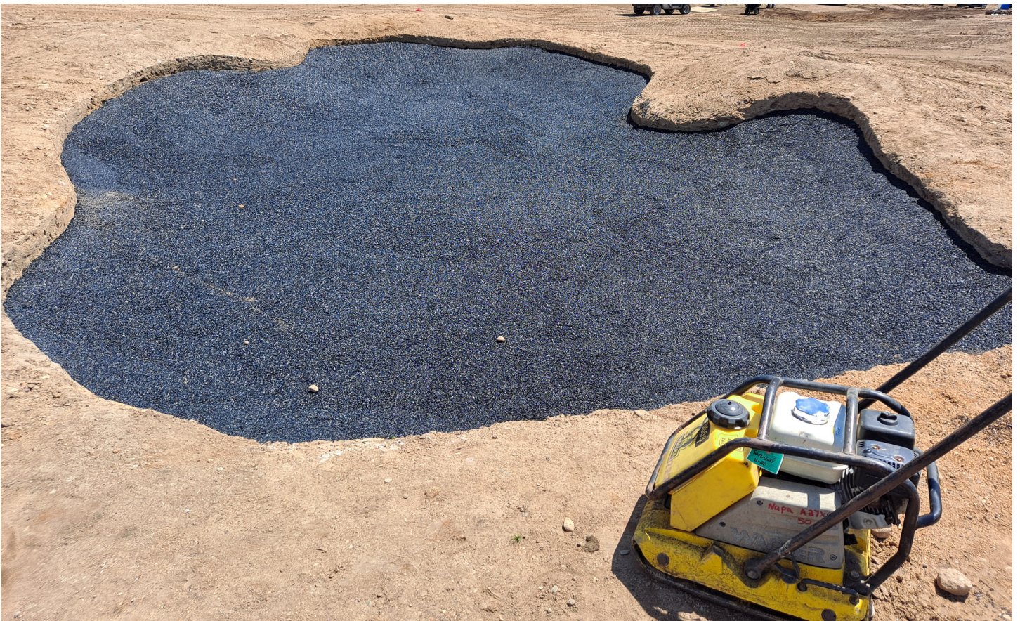
White Course # 1 remodel with new Sand Guard bunker liner. Plate compactor is not for the liner.
