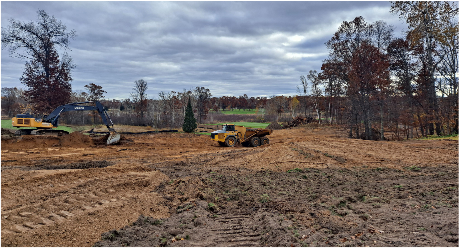
Above: Blue Course #6 New hole ties into the green you see in picture Left: Lehman Course #4 new green/hole
