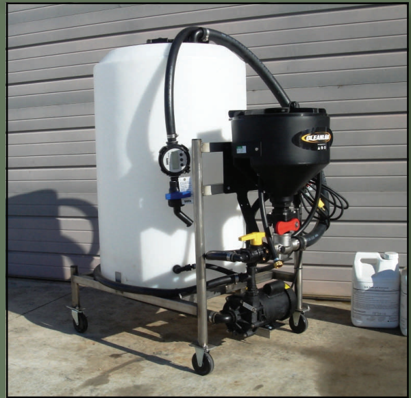
Chemical Pre-mix Station
