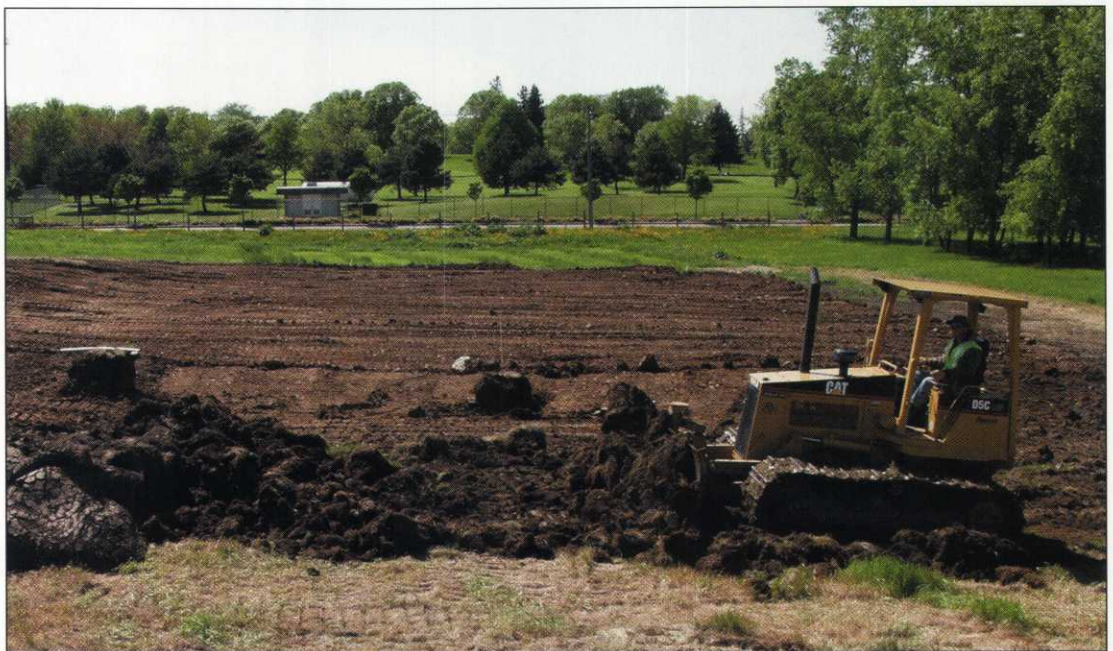
Kentucky Bluegrass Runoff Facility at the University of Minnesota's TROE Center
