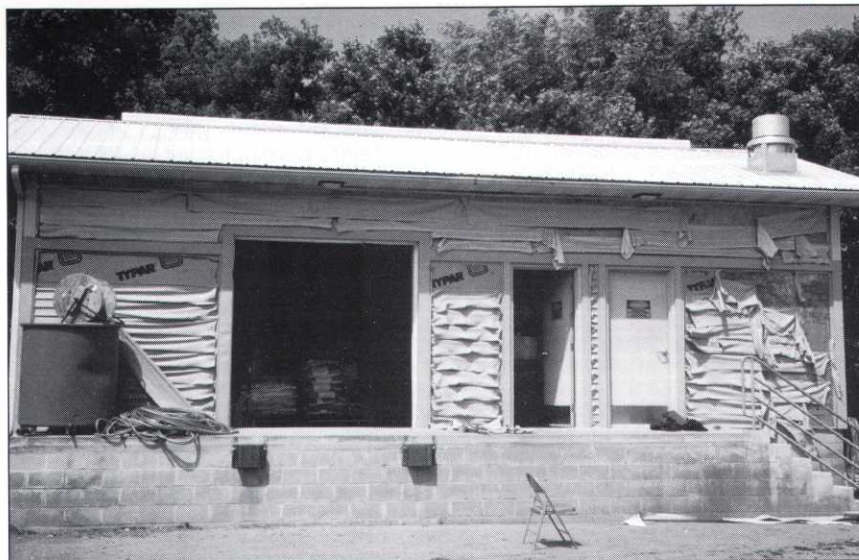
THE CHEMICAL BUILDING AT THE CHASKA TOWN COURSE was spared of any interior damage but the radiant heat from the maintenance building fire caused some exterior damage.
