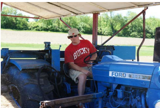
Fig 2. A commercial sod cutter was used to speed the process of removing 15,000 sq feet of sod to start with a fresh base for the Rust Project.
