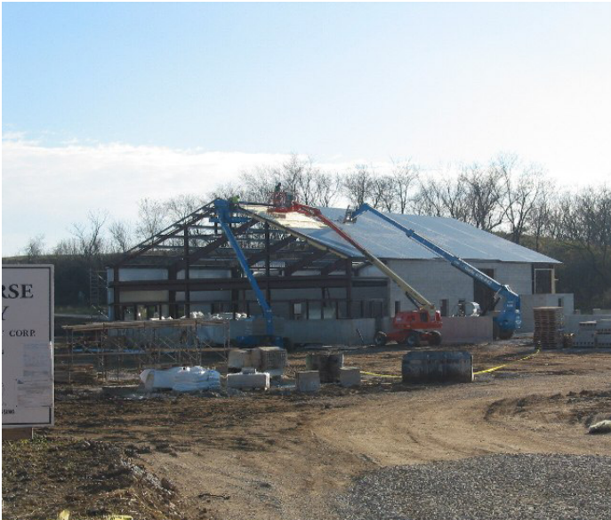
Construction on the new turfgrass facility at Erin Hills was well underway in October.
