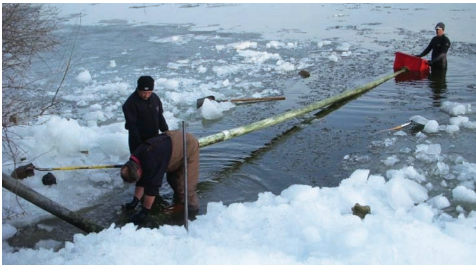
The challenge of starting the irrigation system with ice on the Lake. Notice Superintendent Chad Grimm takes the deep end.
