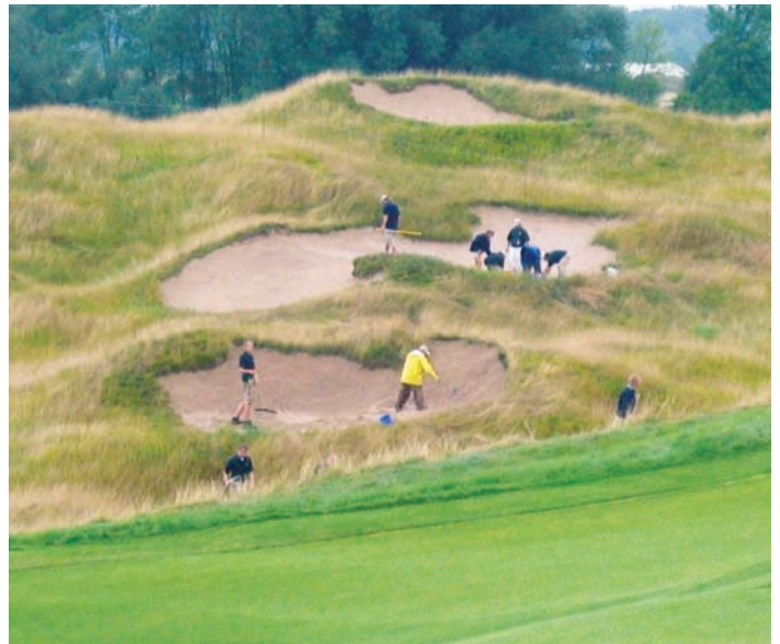
A small group of the bunker crew works on hole 10 with buckets, shovels and rakes.
