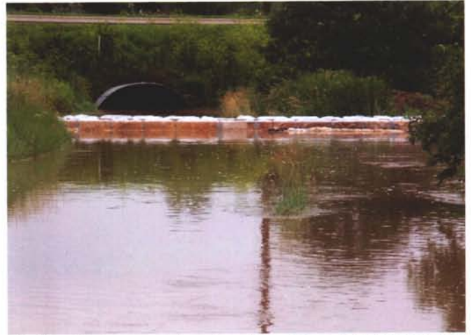
The flood that occurred the day after pouring the piers and deck support beams
