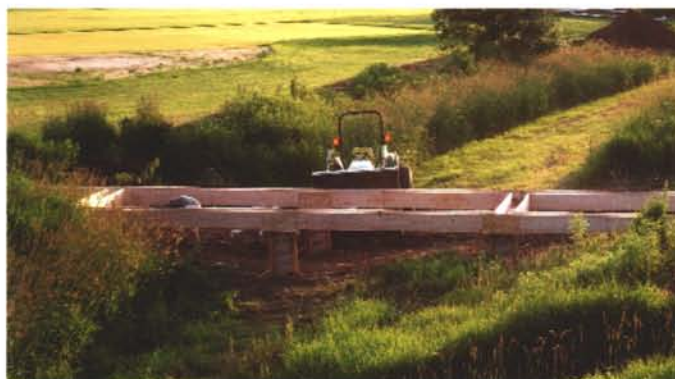
Forms were constructed for pouring the concrete piers and deck support beams
