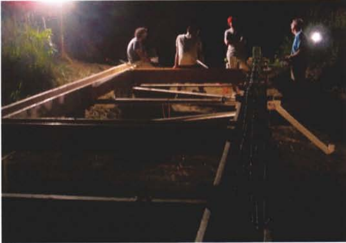
The crew working through the night to tie reinforcing steel bar before the concrete arrives the next morning
