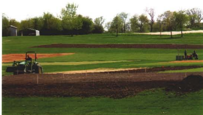
Two new putting greens that were built by grad student Ben Pease will soon have structures installed over them to study growing greens in the shade.
