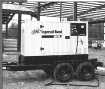
Generators from G20 to G575
