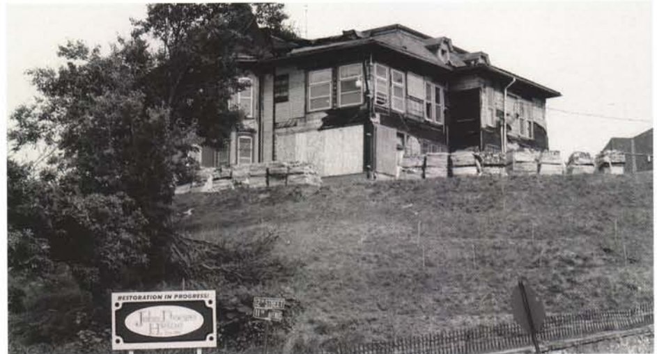
John Deere's home at the corner of 11th Avenue and 12th Street in Moline. It is undergoing an overhaul.
